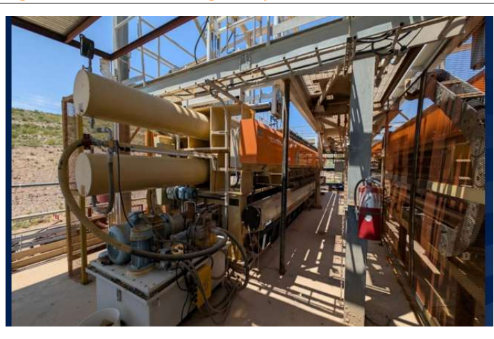
Figure 12: Shafter Processing Facility Filter Press
