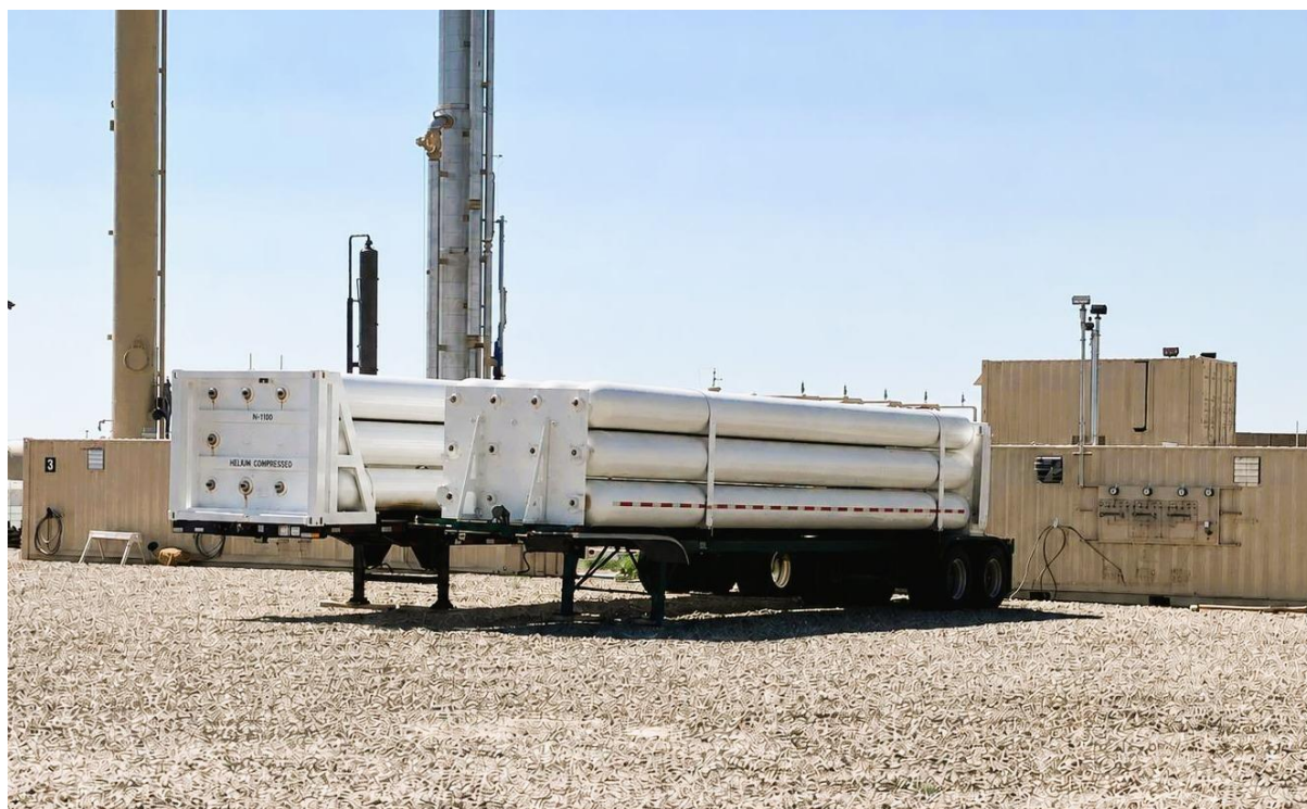
Figure 1: Tube trailers at Pinon Canyon plant
