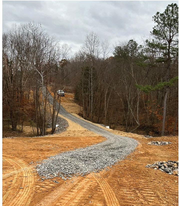
Upgrade of a timber haul road on our Glawson property in Culpeper County, Virginia to access future real estate lot sales.
