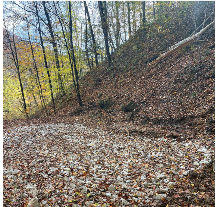
Reclamation site of an abandoned gas well on our Courtney Minerals tract located in Boone County, West Virginia.
