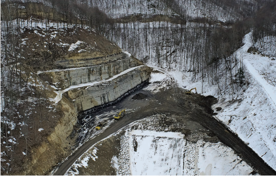
A closer look at the active construction of the new mine portal site on the Powellton Minerals tract.
