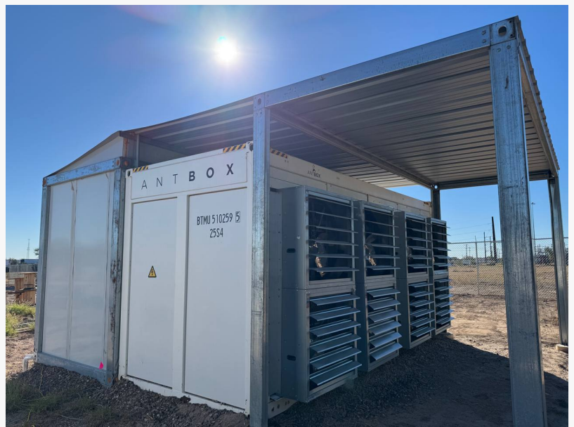
Custom Antbox Cooling System
