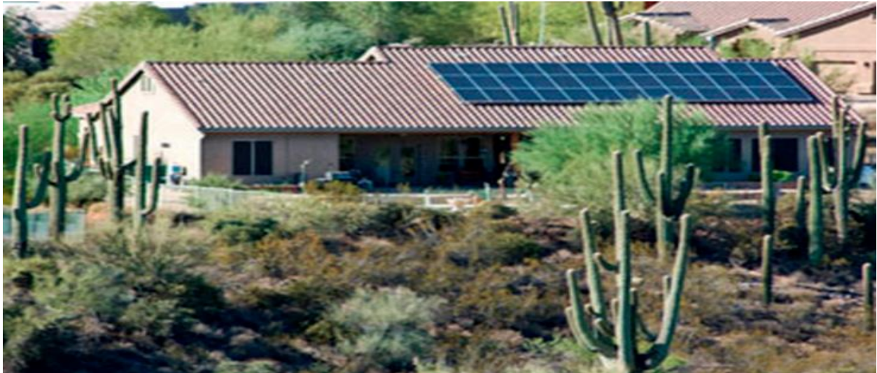
A Typical Arizona Residential solar project
