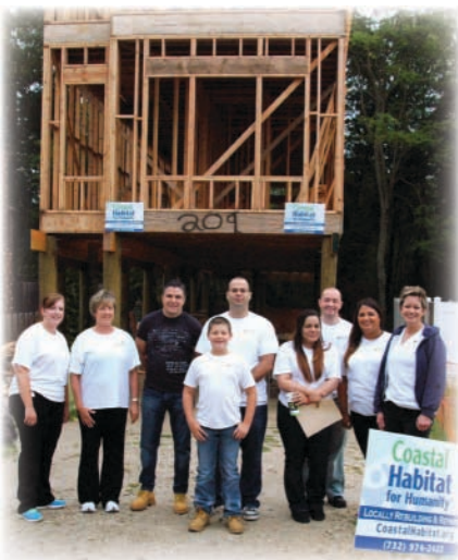
Coastal Habitat for Humanity - Rebuilding a house destroyed by Super Storm Sandy in Neptune, NJ
