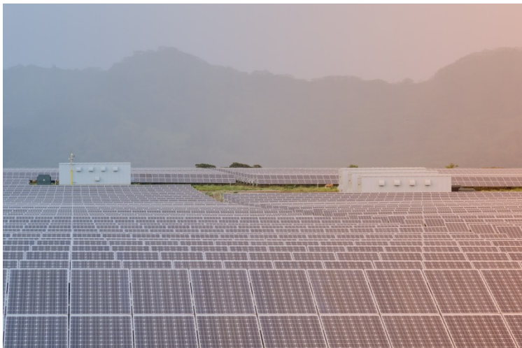
Rows of solar panels in Kauai, Hawaii, where Tesla built a solar-plus-storage project
