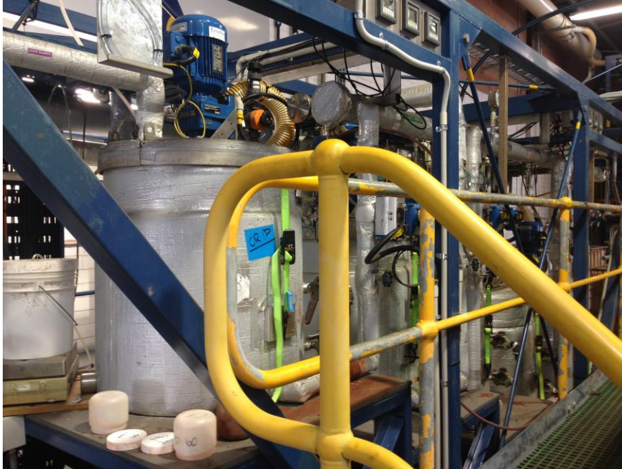
Figure 4: Clean TeQ Pilot Plant: Leached Pulp Neutralisation Circuit
