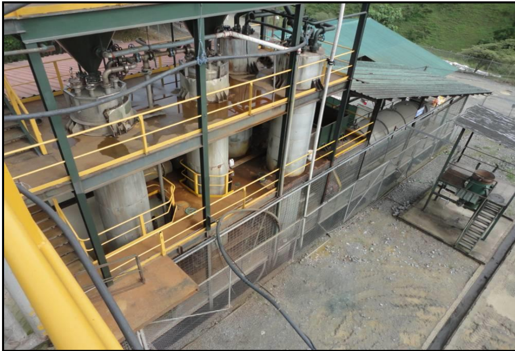
Figure 81: Carbon Desorption and Regeneration Plant.
