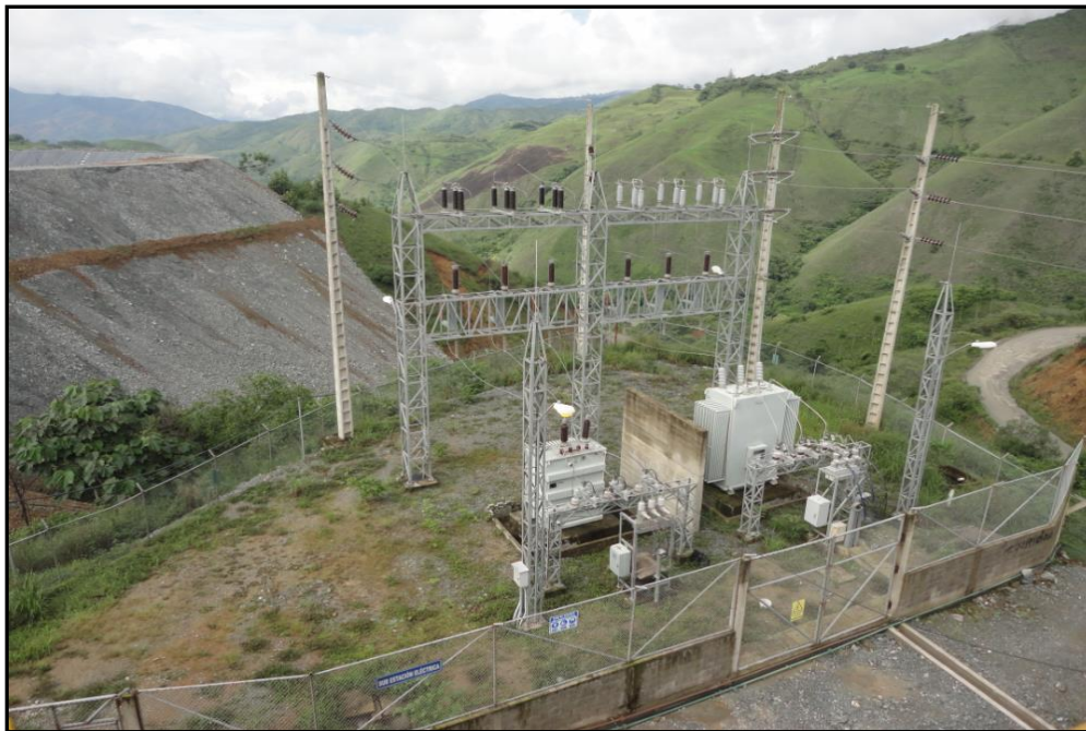
Figure 83: Switchyard 69,000 kV / 420 V (5 MW) and 69,000 kV / 13,800 V (2.5 MW).
