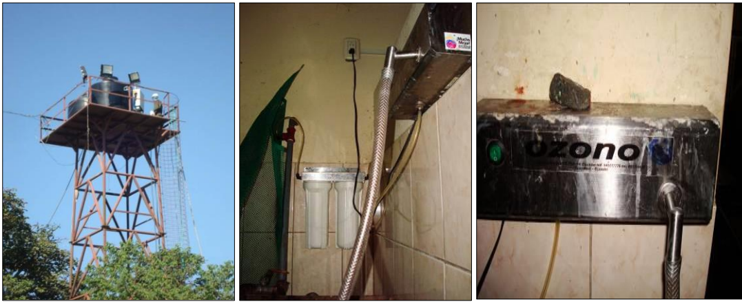
Figure 87: Elevated Water Tanks & Ozone Purification System.
