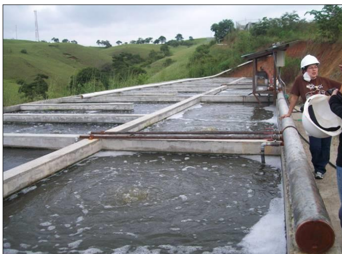
Figure 86: Black and Grey Water Treatment Plant.
