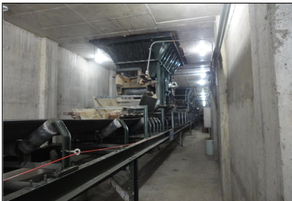
Figure 76: Fine Material Reclaim Feeders.
