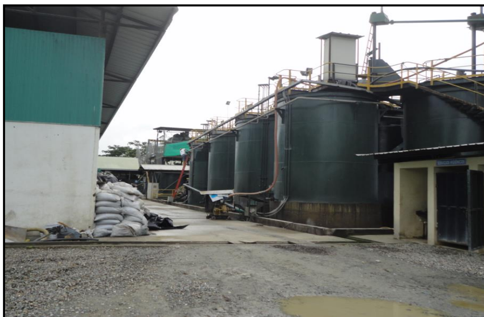
Figure 79: Leaching Circuit Tanks (4 off).
